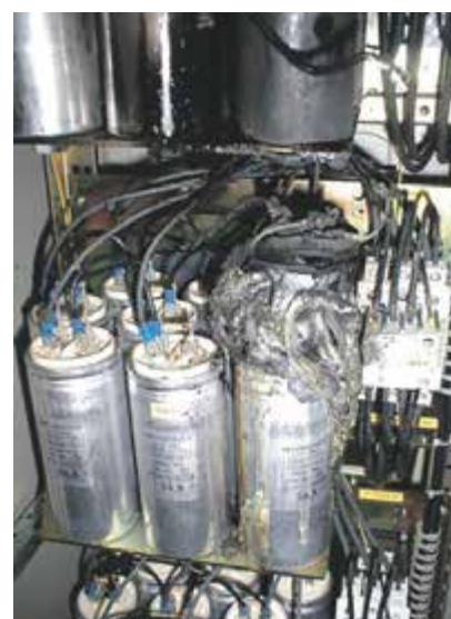
Fig.: Capacitors destroyed by harmonics current
