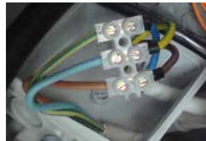
Fig. 7: Here N and PE have been reversed
