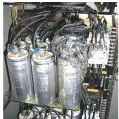
Fig. 6: Destroyed PP reactive power compensation capacitor: A creeping high-impedance ground fault has led to the complete melting of the capacitor and a localized fire.
